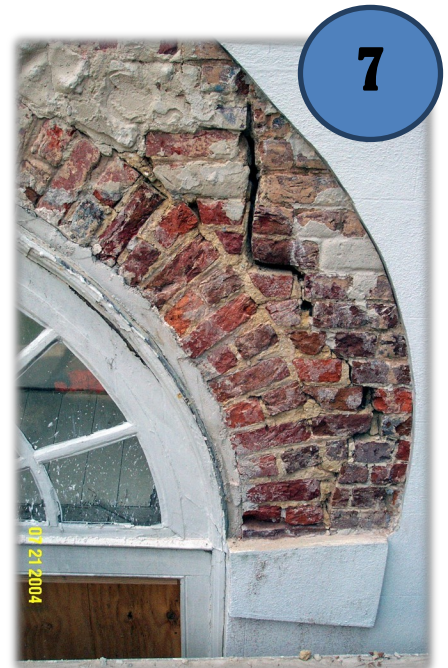
Brick under stucco, 2004 repairs on the west wall; courtesy of Richard Marks Restorations and Old St. Andrew's.
