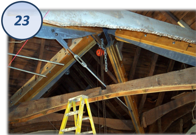
New rafter and collar tie arrangement; courtesy of Richard Marks Restorations and Old St. Andrew's.
