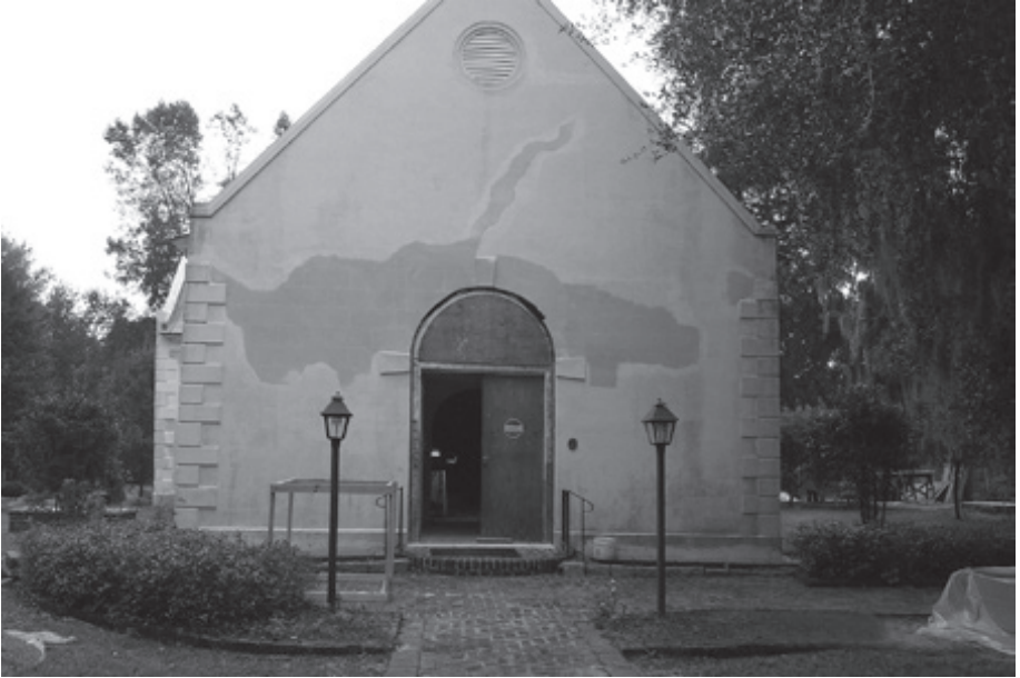
Repairing cracks in the west exterior wall (Courtesy of Richard Marks Restorations and St. Andrew's Parish Church)
