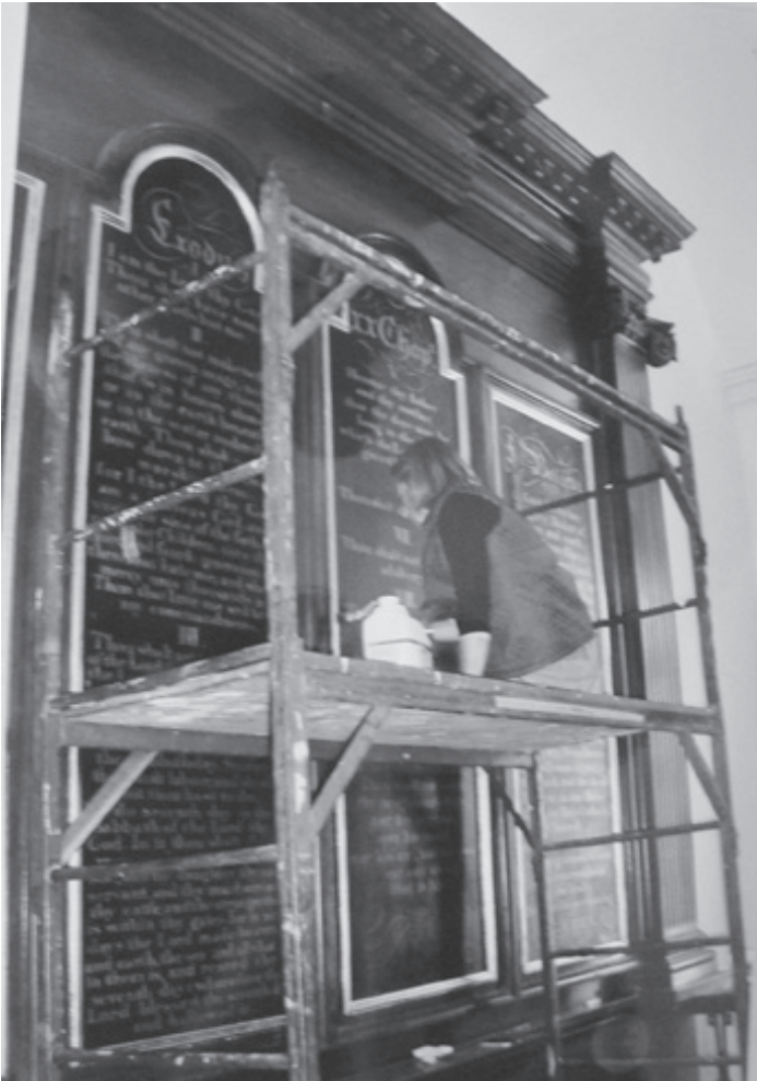
Restoring the reredos (Courtesy of Richard Marks Restorations and St. Andrew's Parish Church)
