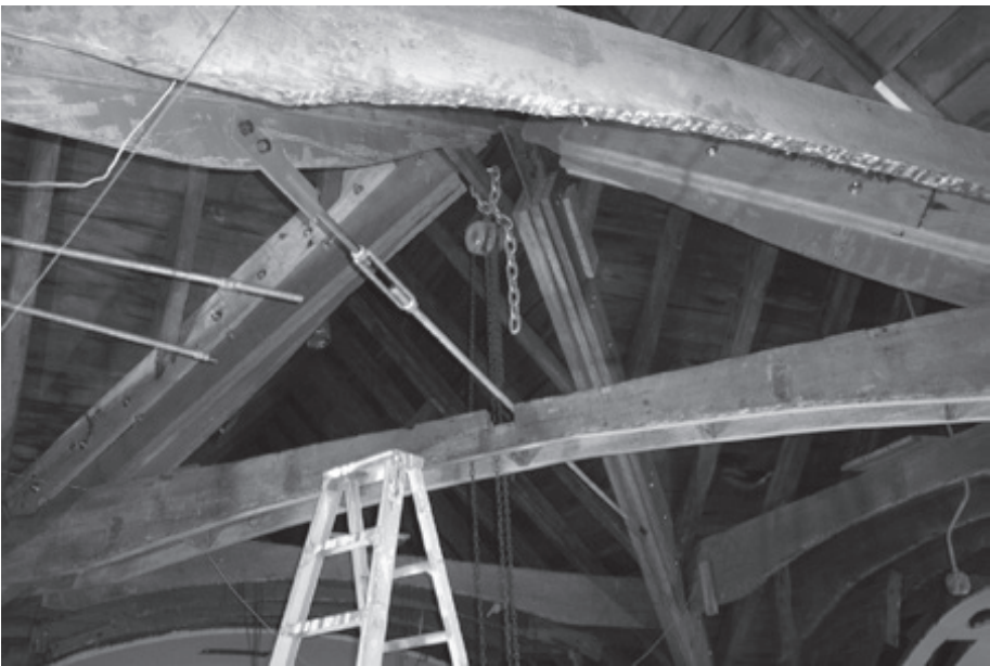
New valley rafter and steel rod collar tie (Courtesy of Richard Marks Restorations and St. Andrew's Parish Church)
